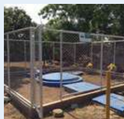
3. Biodigestor reactor biogás
